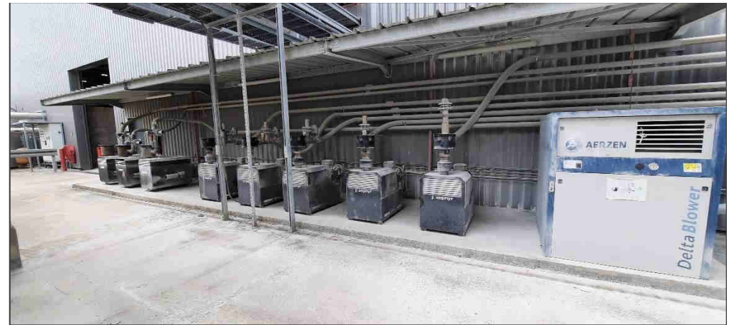
Zone turbines – Pt 22
